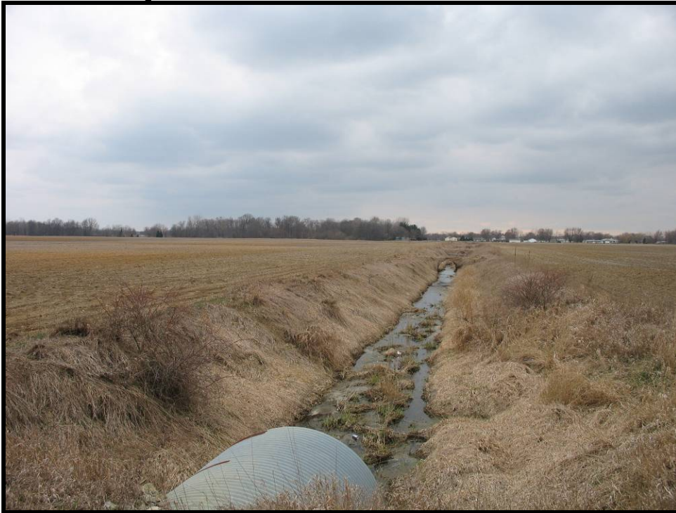
Narrow buffer strip adjacent to Launer Ditch (tributary to Dillon Creek).
