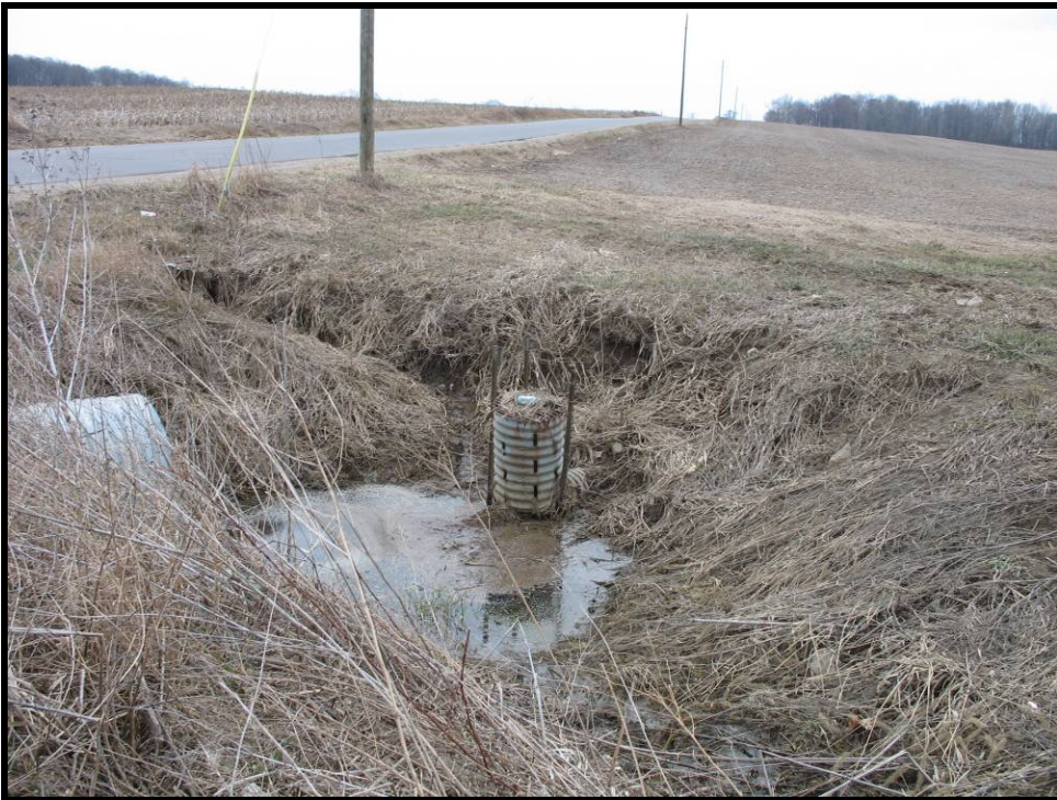
Erosion around tile lines in Dillon Creek Headwaters.
