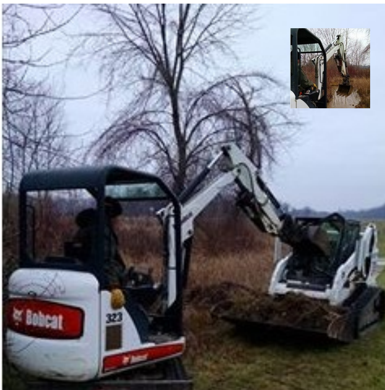
Facing south, removing soil from fish hatchery pond that was parallel to the dam.
