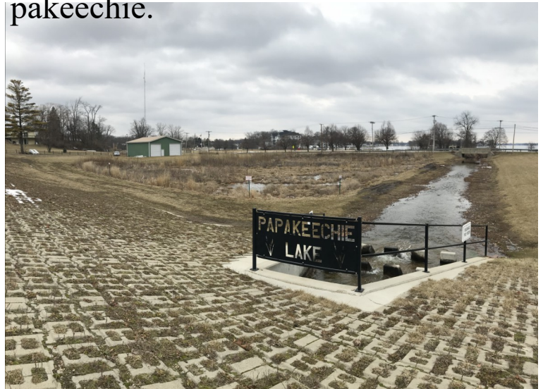
Square pattern is the iron clad flex erosion control mat. This picture is in reverse to be able to read the Papakeechee Lake sign.
