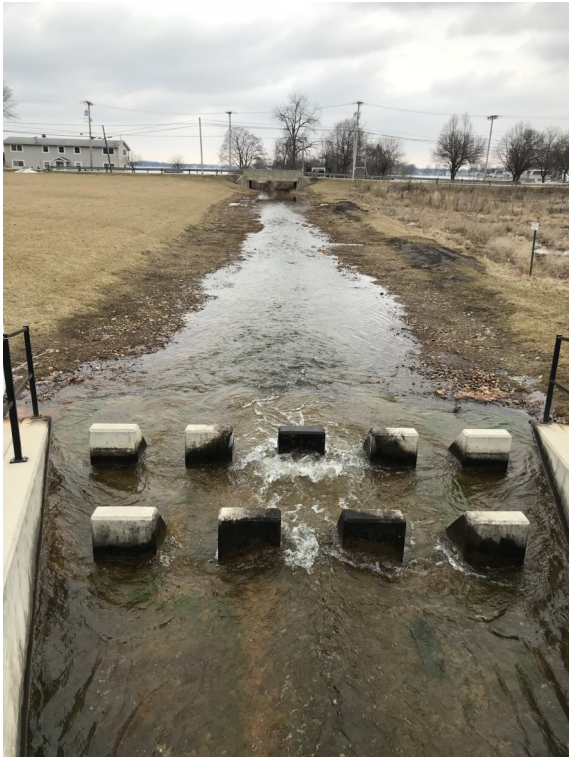
Buffers, diffuser in channel which leads to Lake Wawasee. Flows under Hatchery Road.
